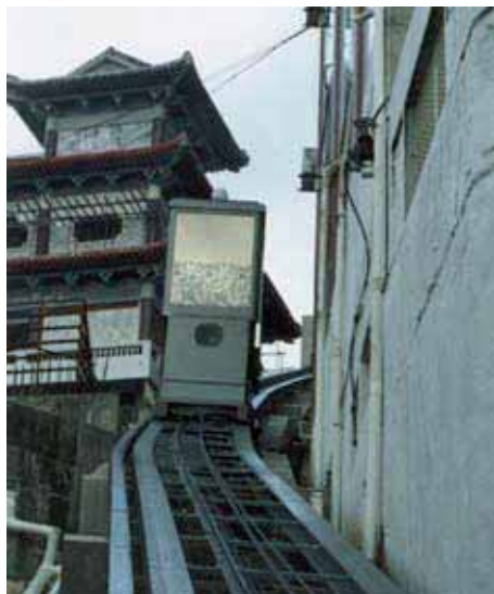
BUDDHIST TEMPLE - MALAYSIA Inclined lift with curved travel Rated load 2250 kg n° 3 stops in line Constant incline 18° Travel 134 m
