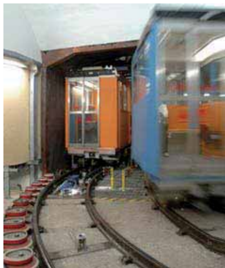
MONTE GALLETTO - GENOVA Automatic lifting system, made of two cars with automatic coupling, with 100 m horizontal travel and 70 m vertical rise, with 1800 kg rated load (each car)
